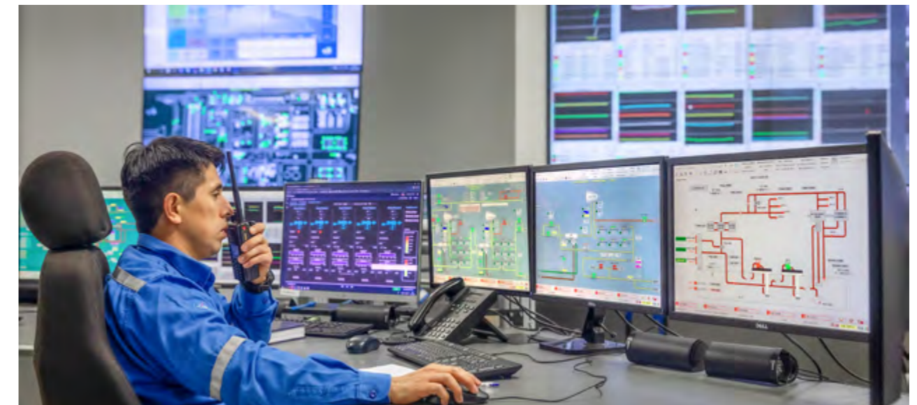
Control Room, Malvinas Plant, Camisea. Peru
